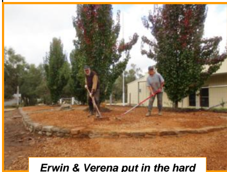
Erwin & Verena put in the hard yakka to build the retaining wall and spread the crushed rock
